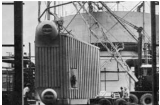
The November 1964 issue of “Fuel for Thought” documented that the system continued to grow quickly after its startup in 1962. Here a new 75,000-lb/hr Combustion Engineers boiler was being installed; the new unit increased steam plant capacity by one-third.
