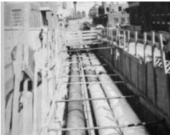
The August-September 1961 issue of “Fuel for Thought” showed the steam and chilled-water pipes being installed down Arch Street toward The Hartford Steam Co.'s new plant.
